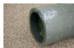
pipes with damaged surface
