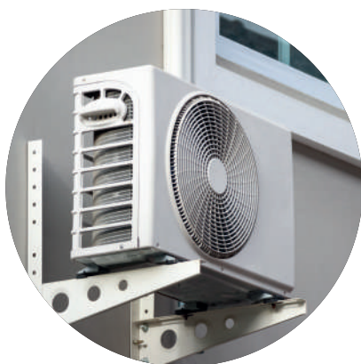
Fixings for air-conditioners
