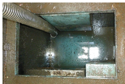
Draining the separator chamber
