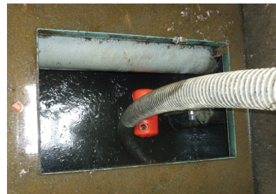
View of the separator chamber
